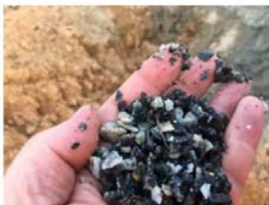
Loose Cuttings Need To Be Removed.
